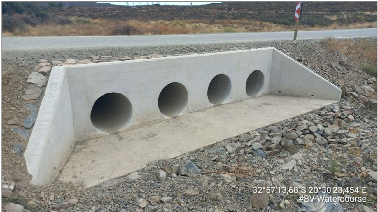
Figure 5: Pipe culvert at road crossing of the Groot River
