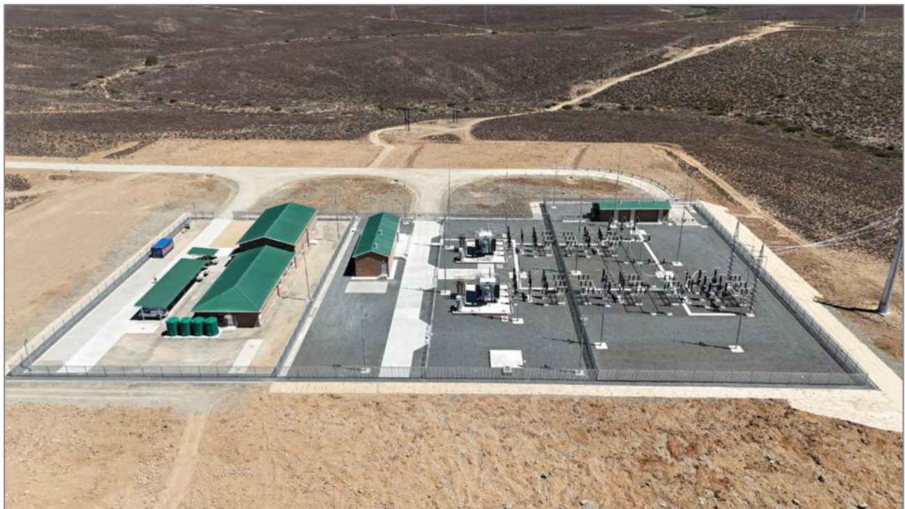
Figure 6: Aerial shot of Brandvalley substation with hessian netting installed
