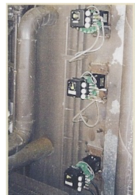
Alstom CE Boiler Windbox. Secondary Air
