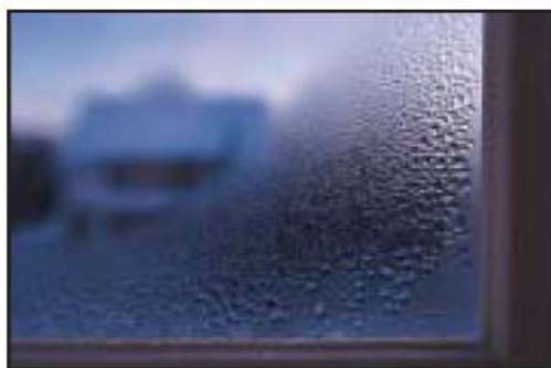
Condensation on the inside of a windowpane.
