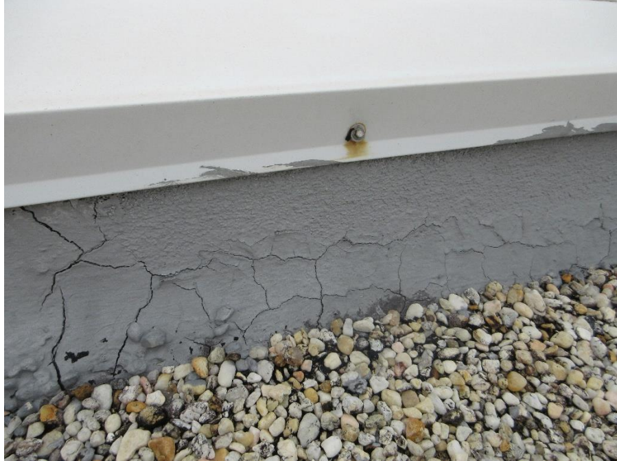
Photo #9 – Loose Fasteners and Scarred Flashing Membrane at Roof Perimeter (TYP.).
