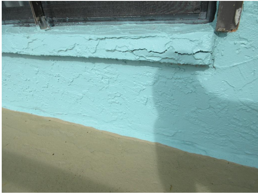
Photo #18 – Broken Windowsill at Unit #501.
