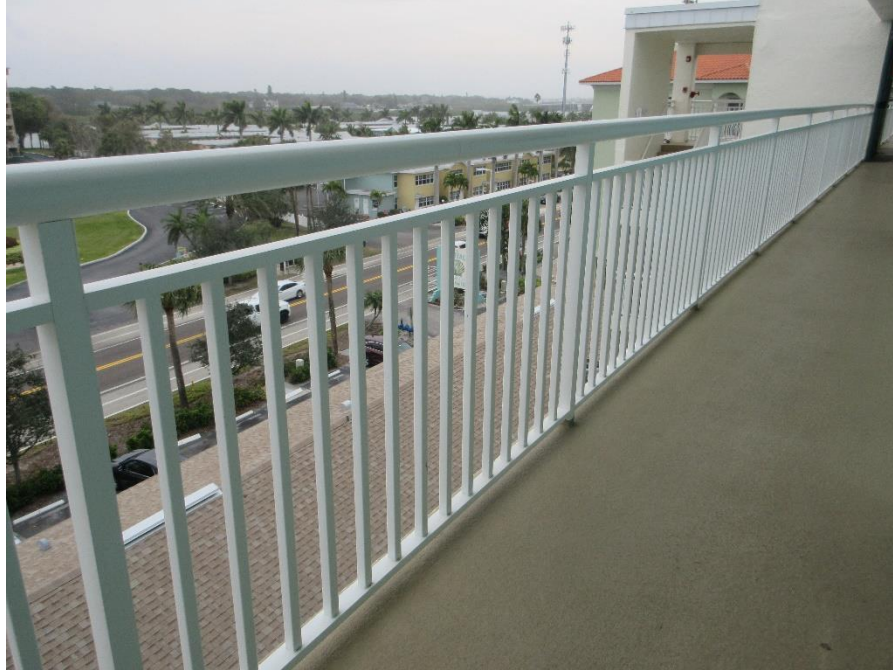
Photo #25 – Typical Balcony Railing at Elevated Walkways (42 ¼" Height, 3 ½" Picket Spacing, 1 ¾" Bottom Rail Height).
