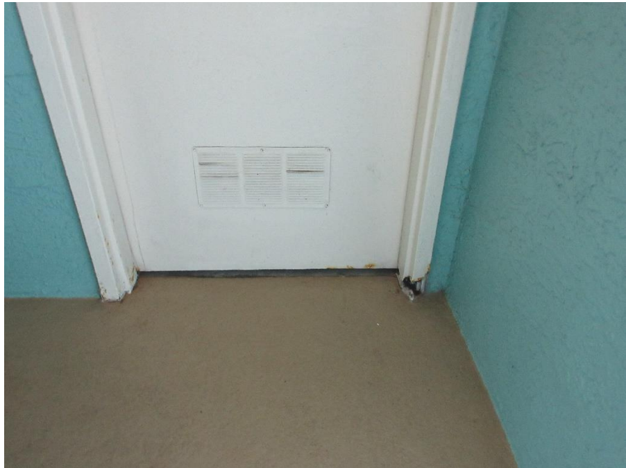
Photo #20 – Corroded Door Jambs at Storage Room (TYP.)
