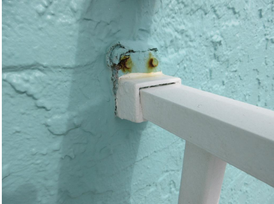
Photo #19 – Broken Railing End Bracket at Walkways due to Rust. (TYP.)
