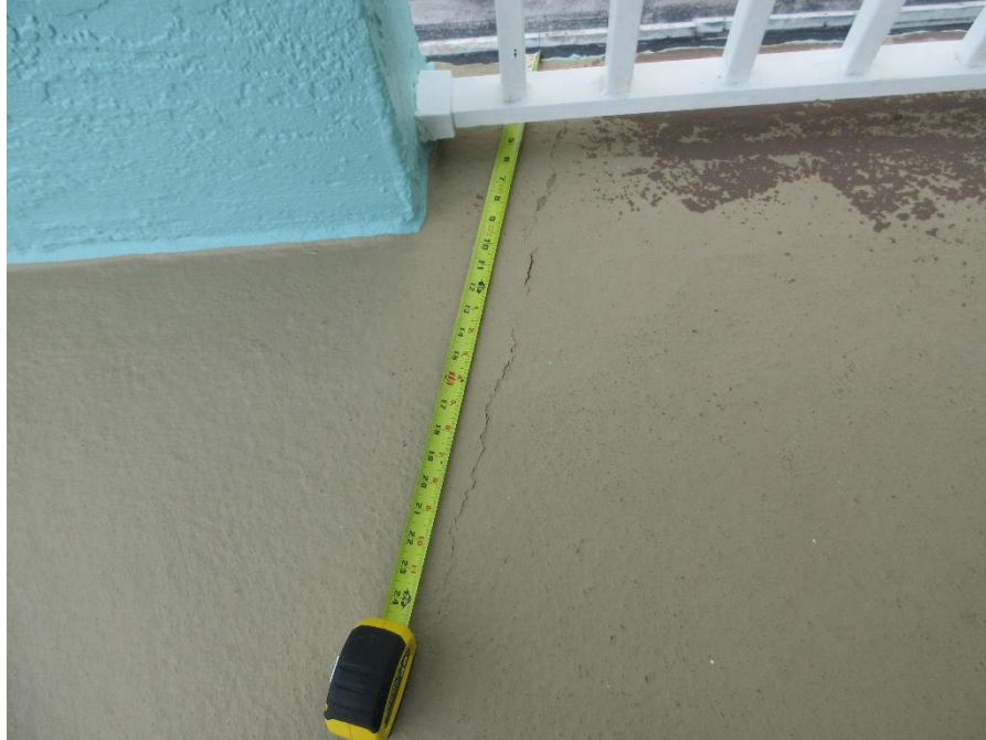
Photo #13 – 45-Degree Crack at NW Edges of Balcony Slabs (TYP.)
