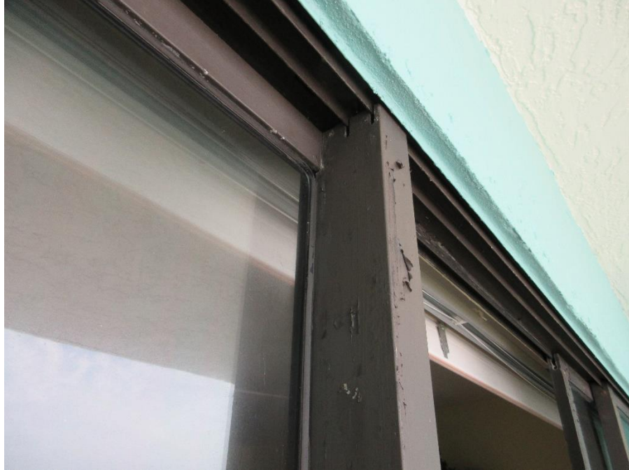
Photo #11 – Peeling Paint at Older Sliding Glass Door (TYP.)
