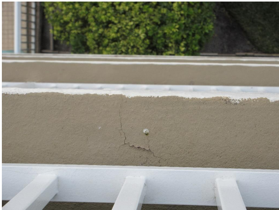
Photo #12 – Hairline Crack Perpendicular to Slab Edges (TYP.)
