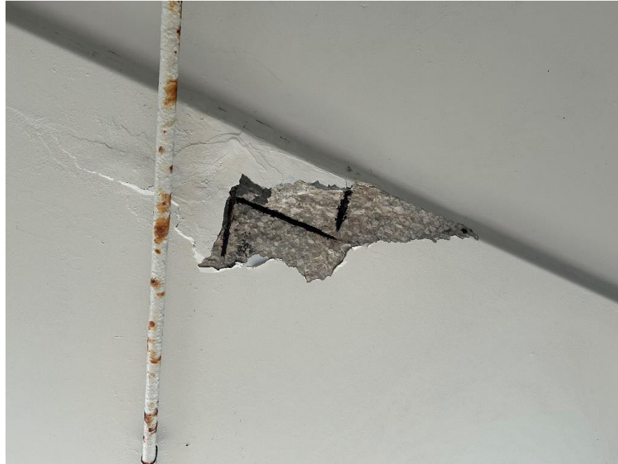
Photo #27 – Concrete Spalls on Underbuilding Parking's Ceiling (TYP.)
