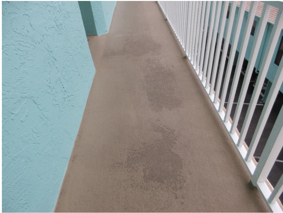
Photo #22 – Typical Concrete Slab Surface Damages or Spalls Covered with Floor Paint (TYP.)
