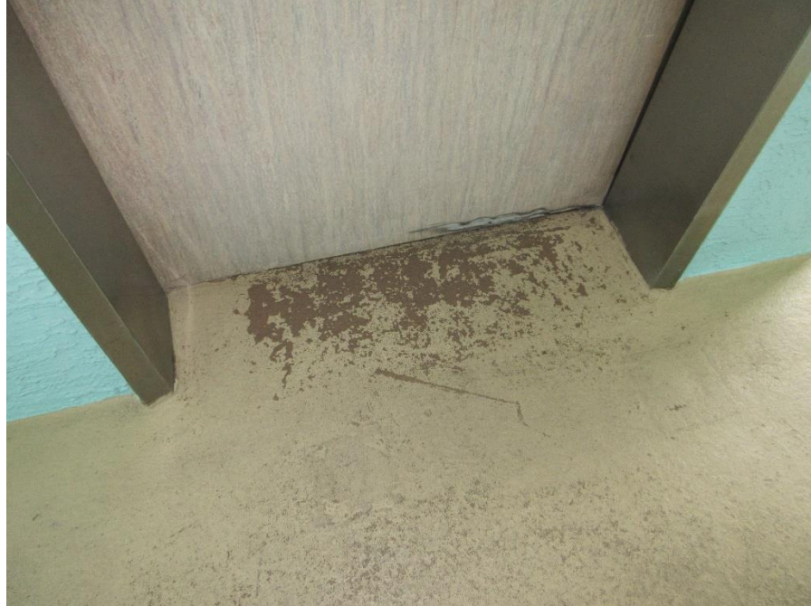
Photo #23 – Deck Coating Peeling at Elevator Room Door (TYP.)
