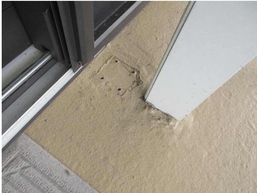
Photo #16 –Unfilled Holes Left in Balcony Deck.
