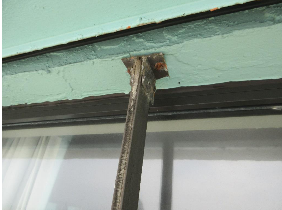
Photo #17 –Corroded Shutters Framing (TYP.)
