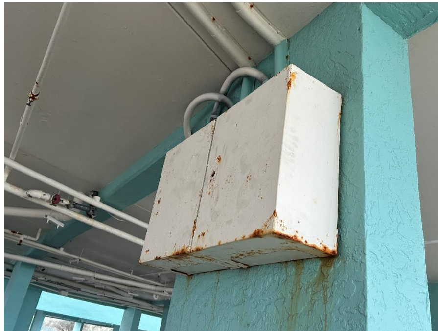
Photo #30 – Rust and Efflorescence at Electrical Meter Box in Garage.
