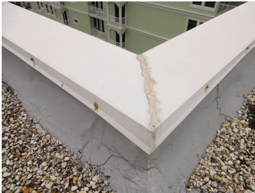
Photo #8 – Rusted Fasteners and failing sealant at Coping Caps (TYP.)
