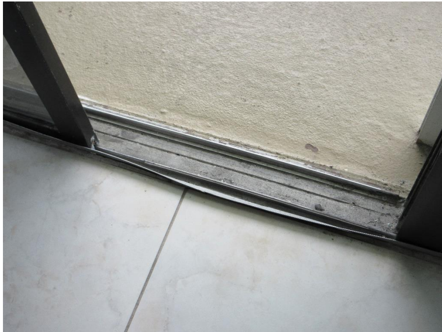
Photo #10 – Damaged and Low Door Threshold (TYP.).
