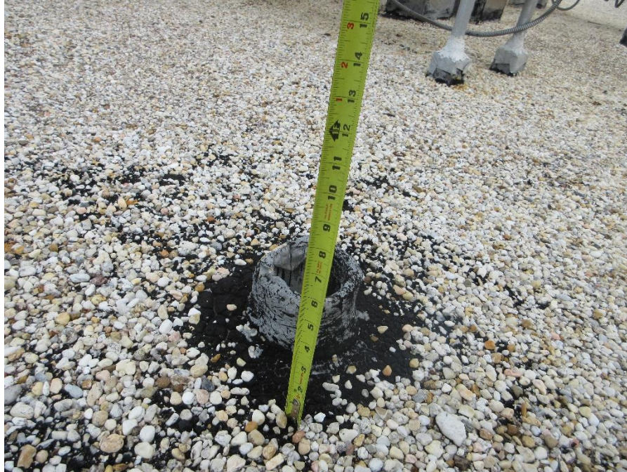
Photo #7 – Roof Vent Pipe Is Shorter than Allowed per FBC.
