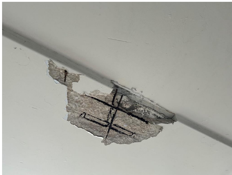
Photo #28 – Concrete Spalls on Underbuilding Parking's Ceiling (TYP.)
