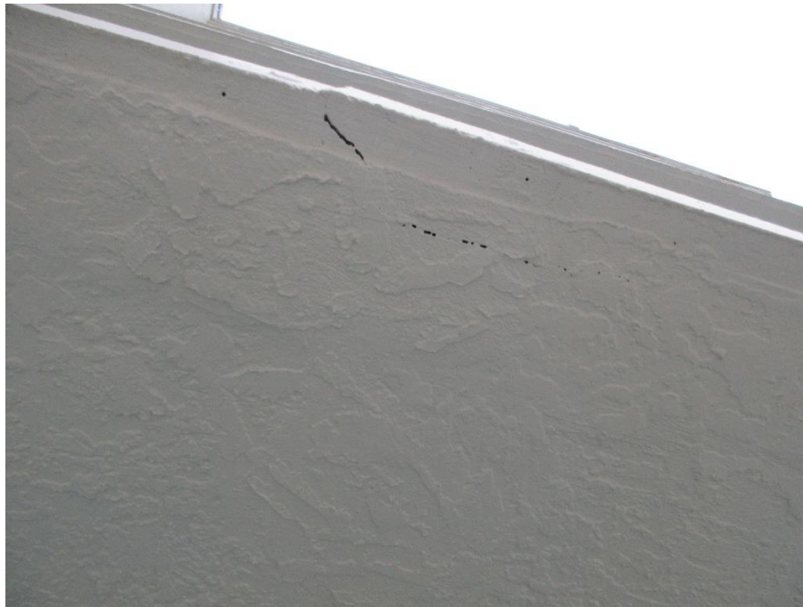
Photo #26 – Concrete Edge Crack at 2 nd Floor Slab on East Side of Building.
