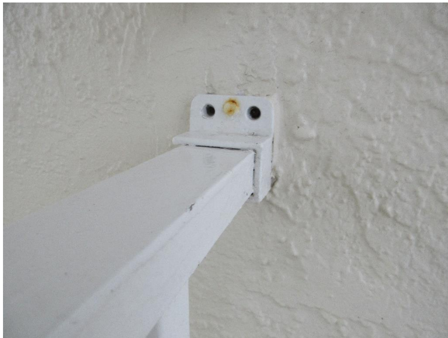
Photo #24 – Missing Fasteners at Railing Ends Brackets (TYP.)
