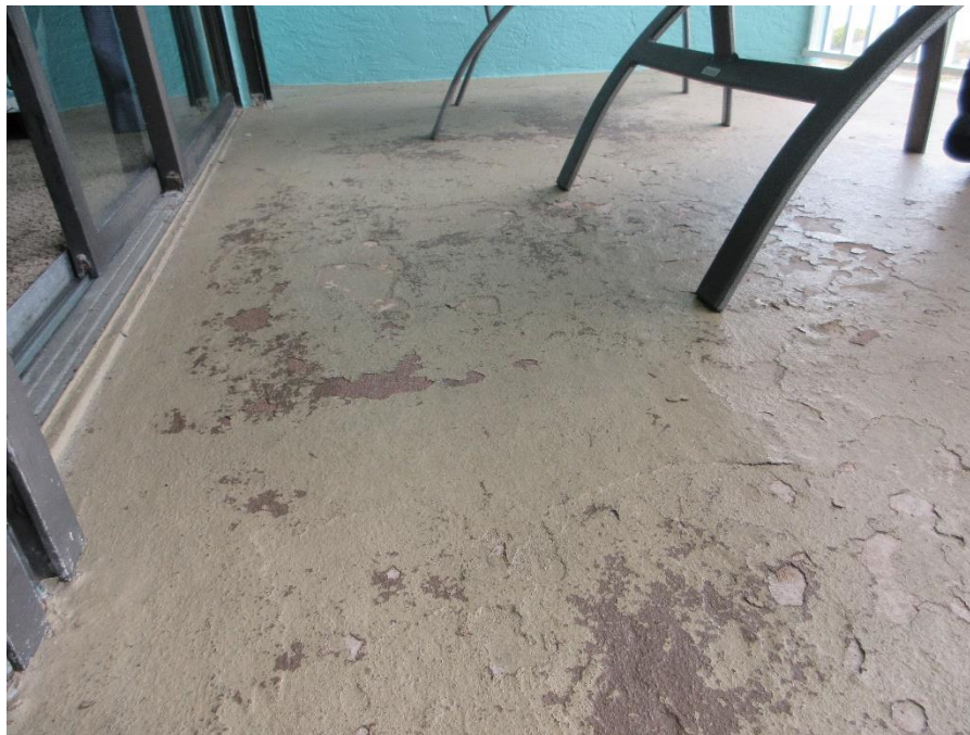
Photo #14 – Deteriorated Deck Membrane at Unit's Balconies (TYP.)
