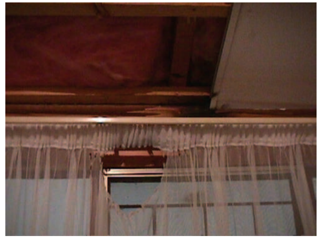
FIGURE 5-21 Damage to curtaining material covering a window of the clubhouse in Figure 5-19. (Copyright Ian R. Jandrell.)
