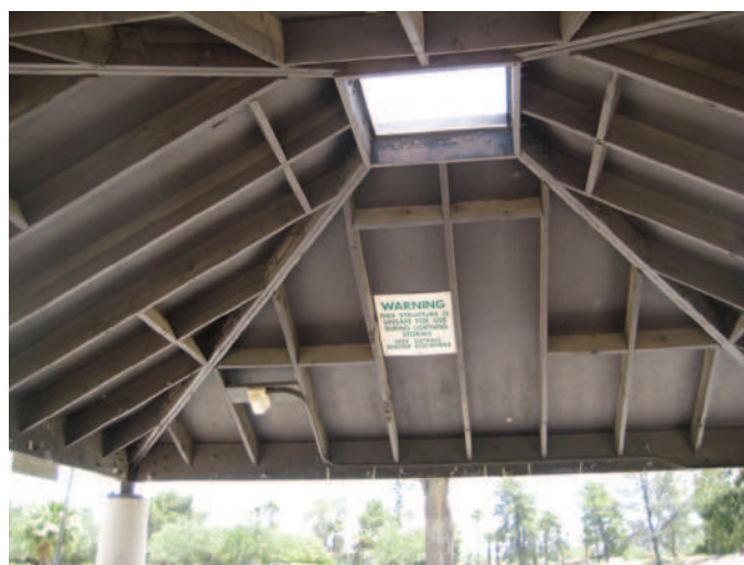
FIGURE 5-47 Lightning-unsafe picnic shelter in Tucson, Arizona. Note warning sign on roof, which states: “WARNING: This structure is unsafe for shelter during lightning storms. Seek suitable shelter elsewhere.”
