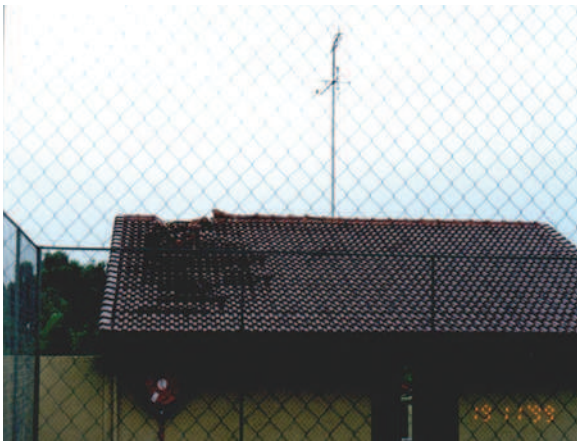
FIGURE 5-19 Damage to the roof of a clubhouse from direct lightning strike. The damage was extensive and included structural damage to the clubhouse. (Copyright Ian R. Jandrell.)
