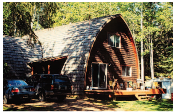
FIGURE 14-13 This permanent residence, located in west-central Alberta, Canada, is unlikely to survive exposure to even a low-intensity wildland fire, and it would be difficult to stay and defend it for a number of reasons. There is dense forest vegetation immediately adjacent to the structure. Cedar shakes have been used for roofing. This has been shown time and time again to be the “kiss of death” in wildland-urban interface fires (at the time this photo was taken in 1997, the shingles were in such bad shape that they had lichens growing on them). The homeowner also liked to store flammable materials under his deck. (Courtesy Yukon Wildland Fire Management; photo by A.K. Beaver.)
