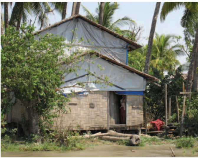
FIGURE 85-20 Plastic sheeting repair to houses after Cyclone Nargis in Burma (Myanmar). (Courtesy Sheila B. Reed.)
