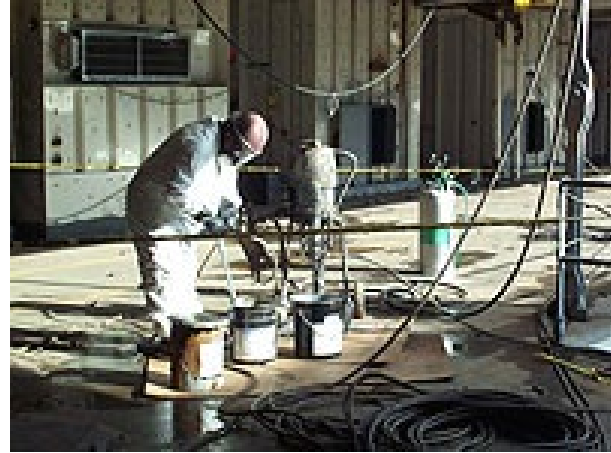
Physical: Paint mixing/spray booths/chemicals
