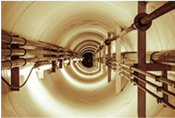
Pipes and pipelines
