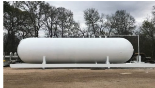
Horizontal Pressurized Tank
