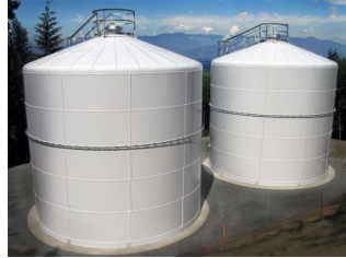
Cone Roof Tank
