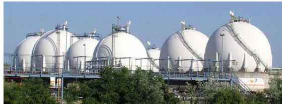
Spherical Pressurized Tank
