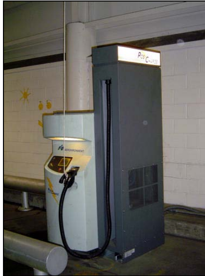
Figure 3-12: EV Fast Charging Station (Photo courtesy of NREL Photographic Information Exchange)
