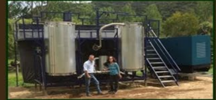
2021 - extraction plant, commissioned/ready
