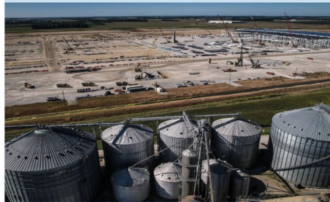
$5B Honda EV Plant being Constructed in Fayette County. Source: Dayton Daily News.
