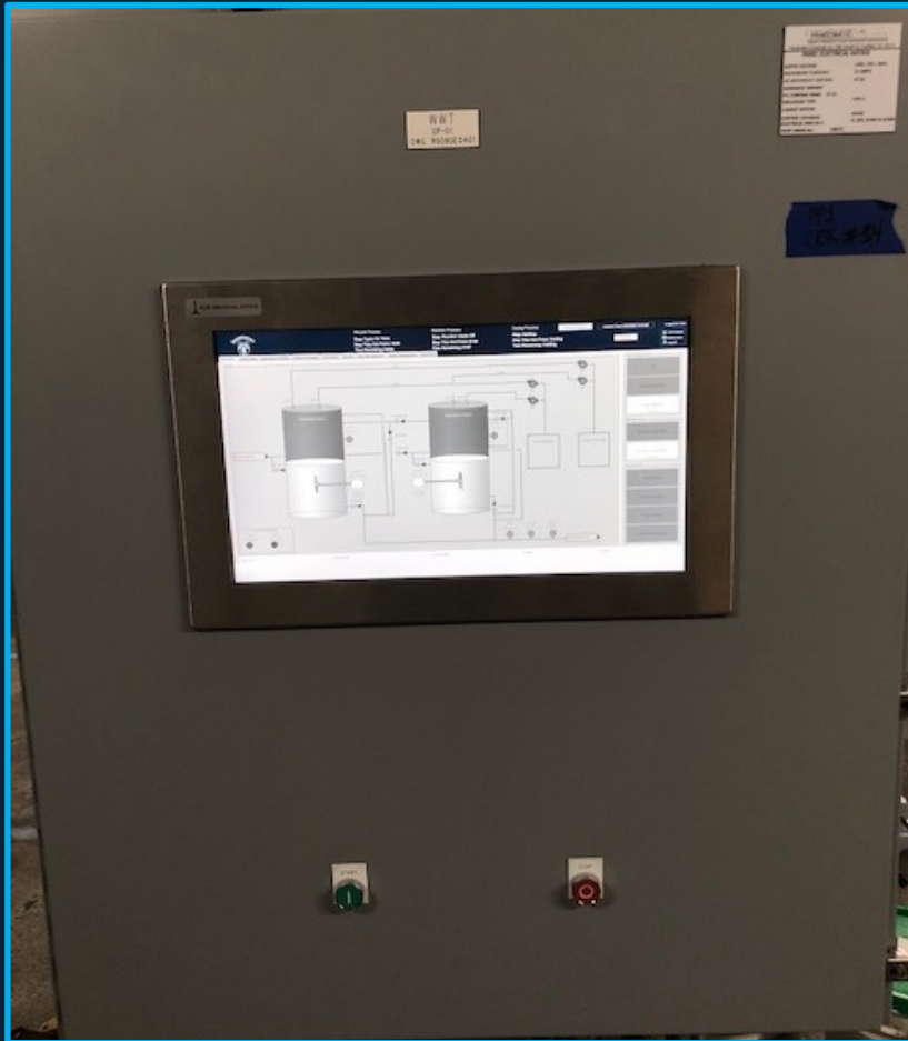
PROGRAMMABLE LOGIC CONTROLLER (PLC)
