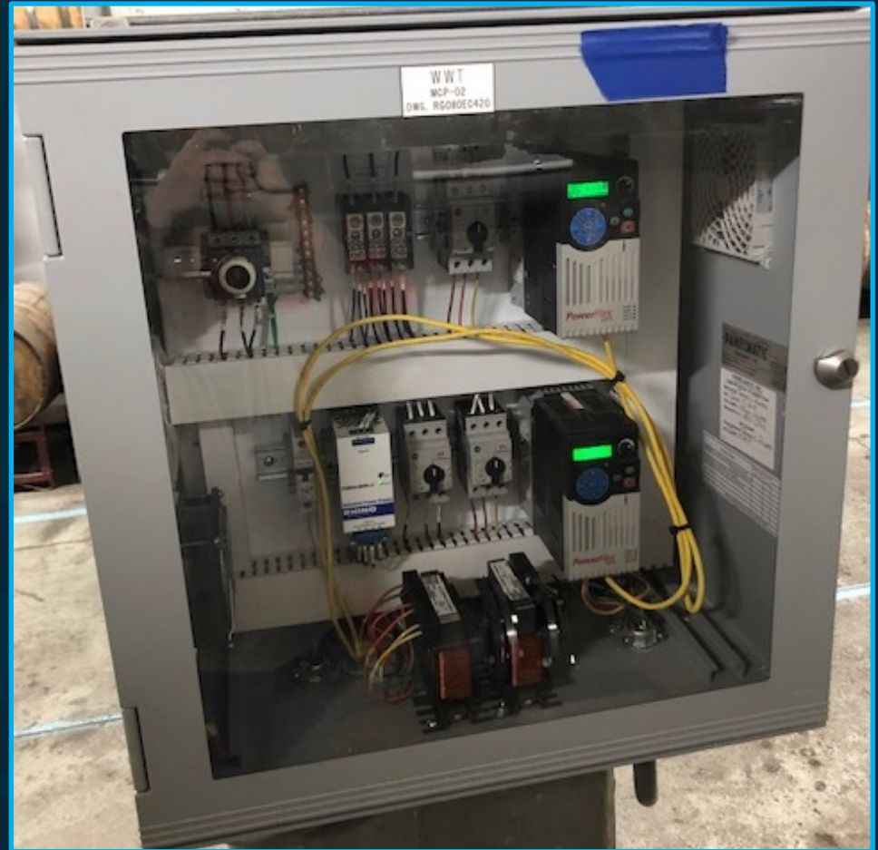
MOTOR CONTROL CENTER
