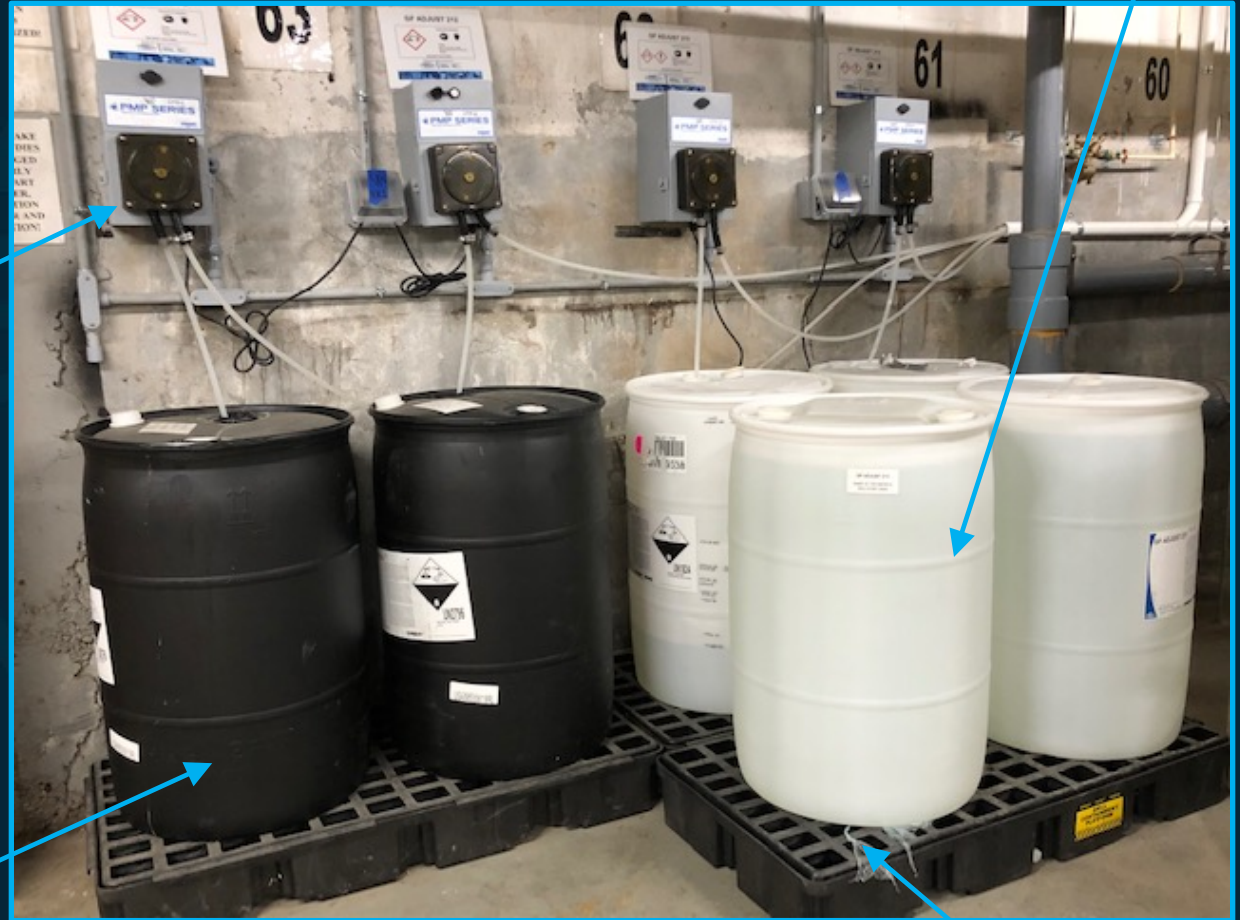
CHEMICAL DOSING PUMP • 4 TOTAL PUMPS
