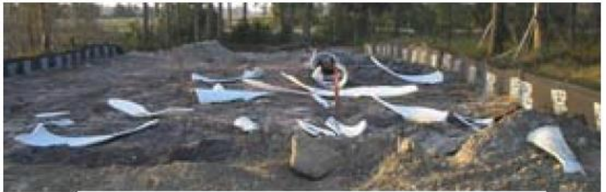
Collier County, FL, fused PVC failure during pressure test.
