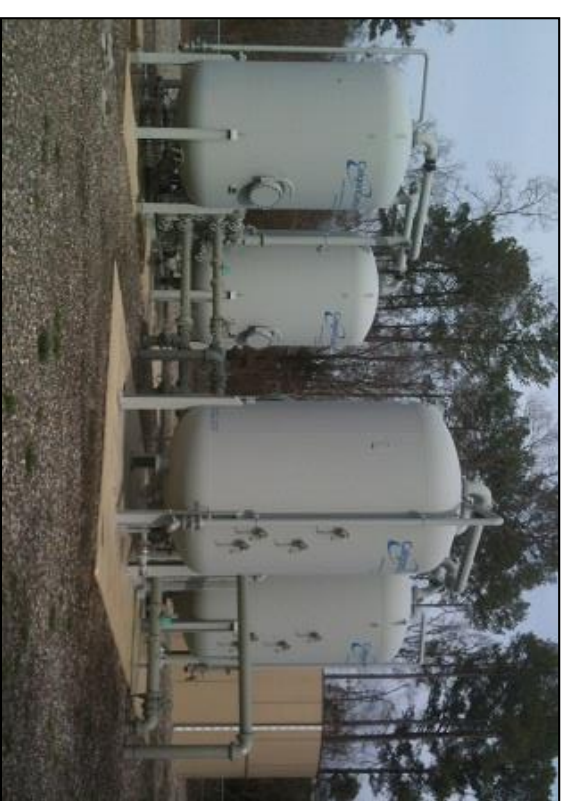
GAC reactors Greater Onachita, Louisiana
