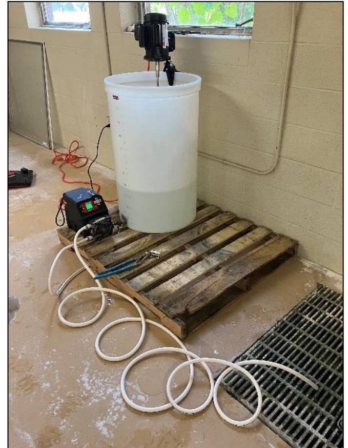
Temporary carbon feed system
