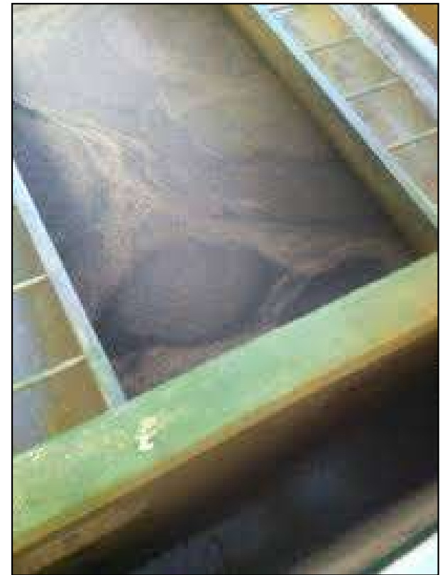
Excess fluidization due to gravel displacement
