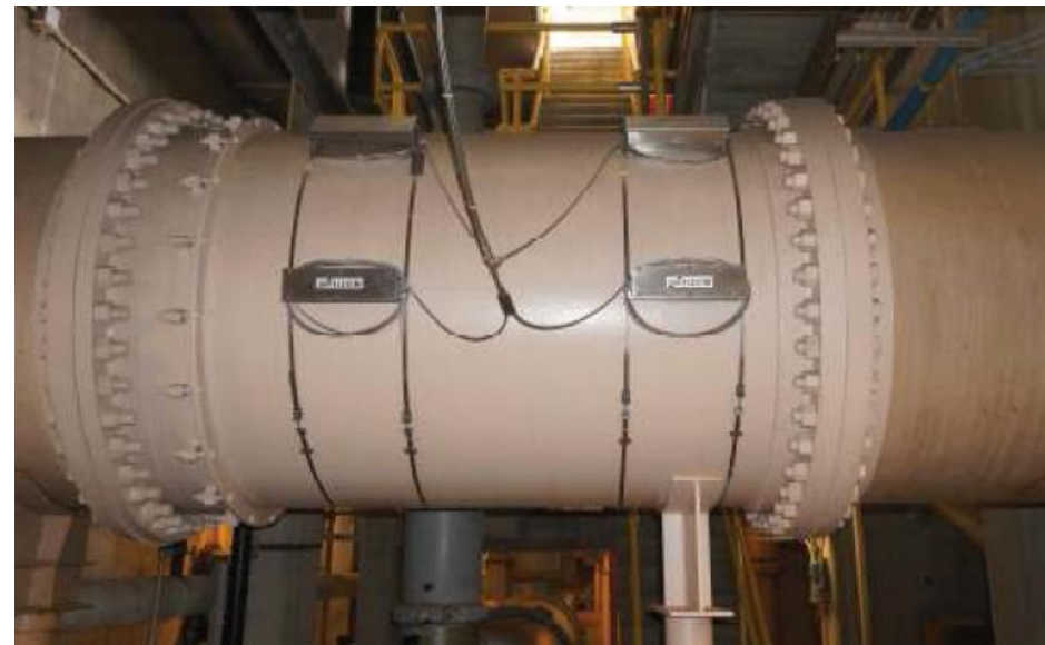
Figure 2: 2path - 4beam Ultrasonic On 48" spool piece
