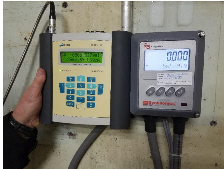
Figure 1: Low Cost Ultrasonic Reading 0.00 GPM. Advanced Technology Reading 2,960 GPM
