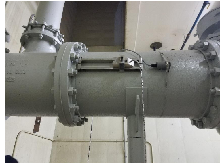
Figure 2: 18" Ductile Iron Line, G Sensor in Direct Mode next to Existing Low Cost Sensor
