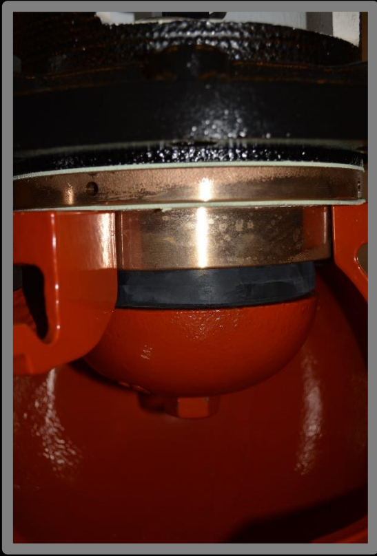
Hydrant Closed Drains Are Open
