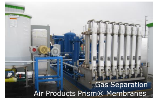
Gas Drying & Compression
