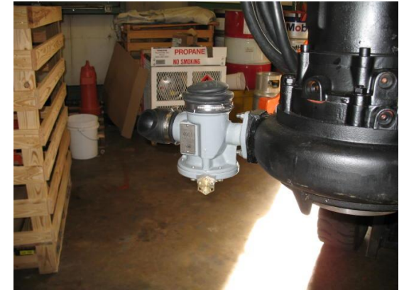
Mix Flush Valve
