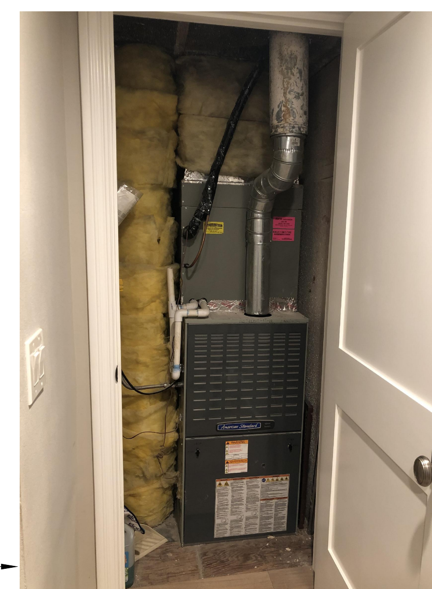
PICTURE OF THE MECHANICAL EQUIPMENTS TO BE RELOCATED, ALL DUCT WORK TO REMAIN THE SAME. FOR REFERENCE
