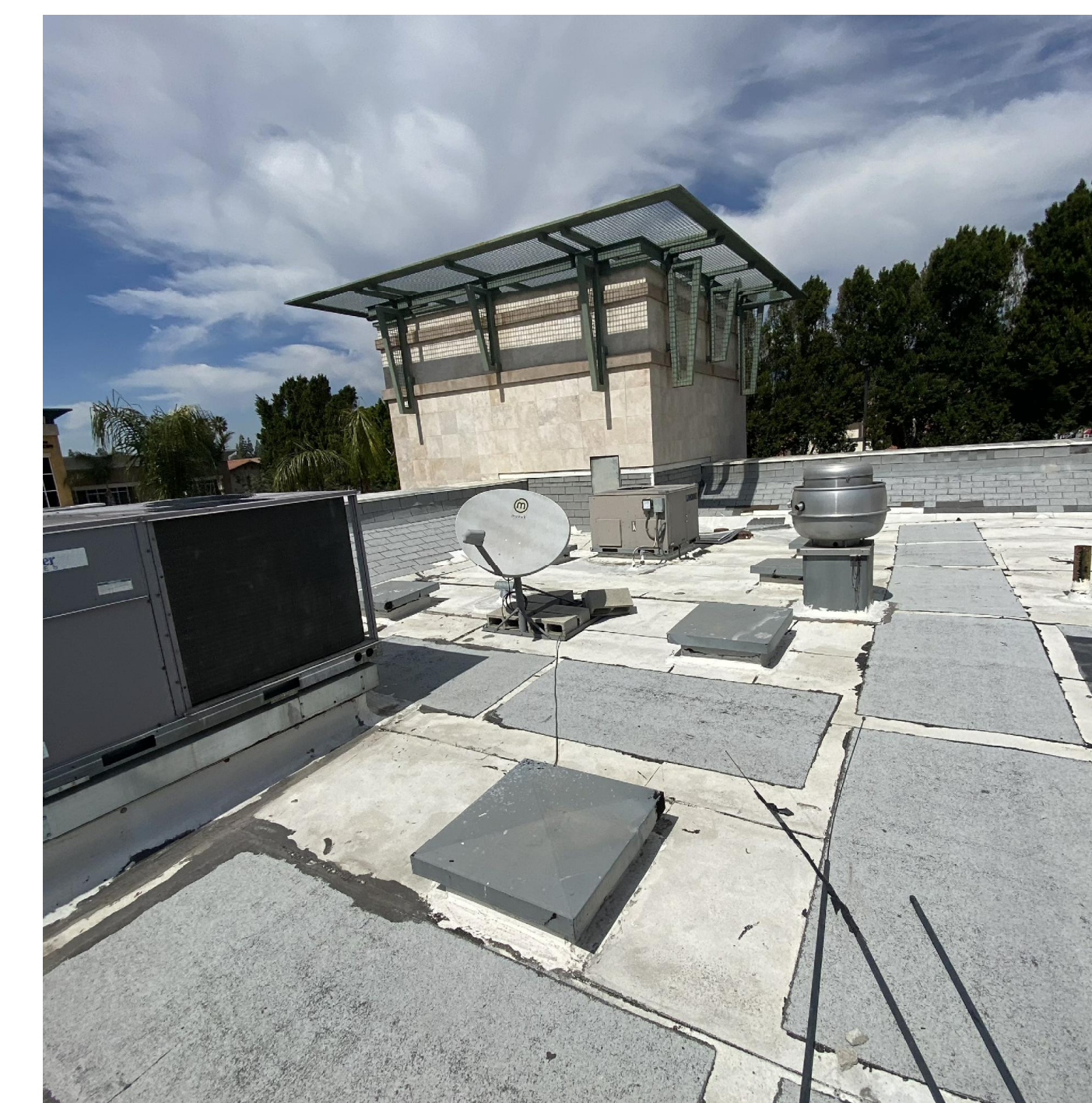
PICTURES SHOWING THE ROOF EXISTING CONDITIONS, NO ROOF PENETRATION NEEDED IN THIS SCOPE OF WORK. ANY ROOF PENETRATION HAS TO BE SUBMITTED TO STRUCTURAL ENGINEER AND STAMPED PRIOR TO COMMENCING OF WORK
