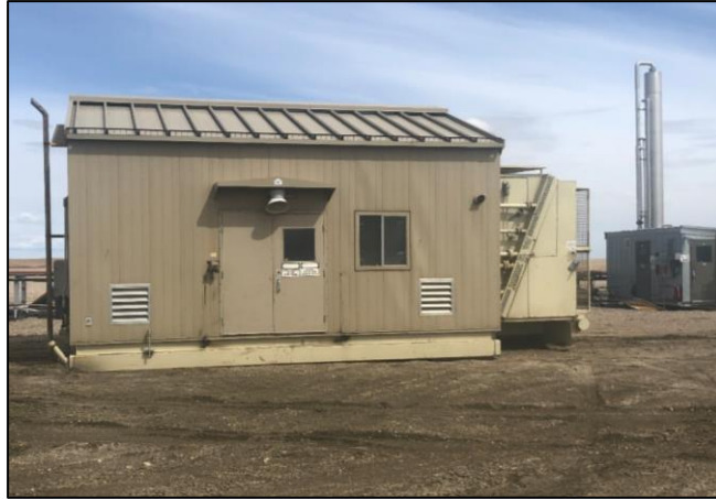
Compressor Site ~1 to 7 days
