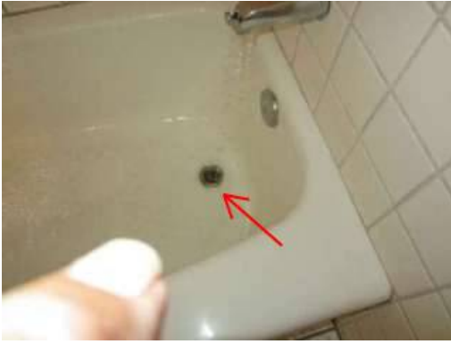
Photo 11-7 The bathtub drain is missing a stop.
