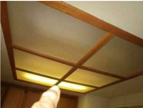
Photo 14-1 The lighting soffit fluorescent bulbs are not working and should be replaced.
