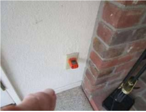
Photo 5-3 The fireplace exterior plug does not work correctly, it is also the wrong outdoor plug per code. A licensed electrician should repair it.
