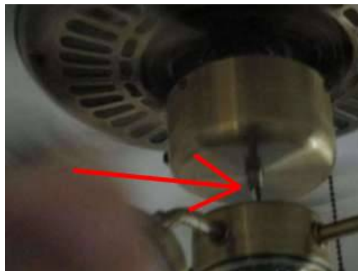
Photo 13-2 The fan in the living space bedroom needs repair. Electrical wires are holding fan from falling this is a safety hazard and issue.
