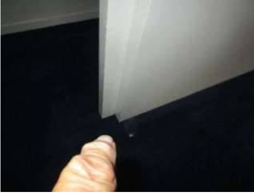
Photo 13-17 The pocket door does not move freely and this should be repaired.
