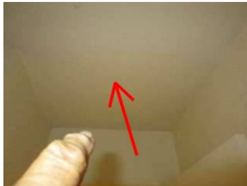
Photo 13-14 Smoke detectors need to be installed in each room. A carbon monoxide detector is missing and needs to be installed.
