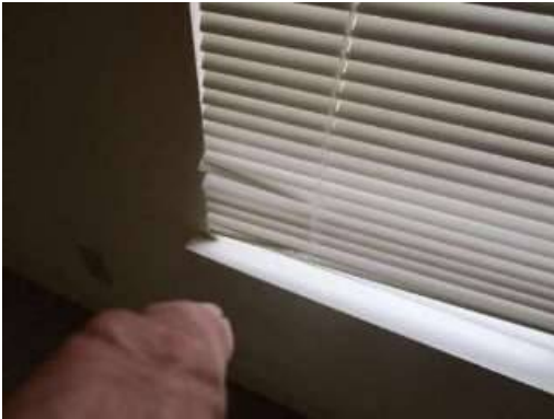
Photo 13-5 The blinds are broken in some areas of the house.
