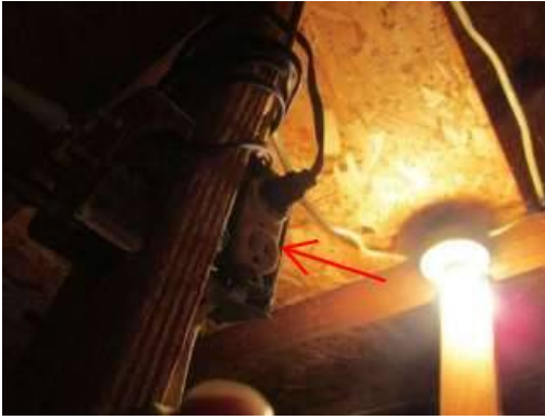
Photo 5-4 The attic electrical outlet needs a cover plate.
