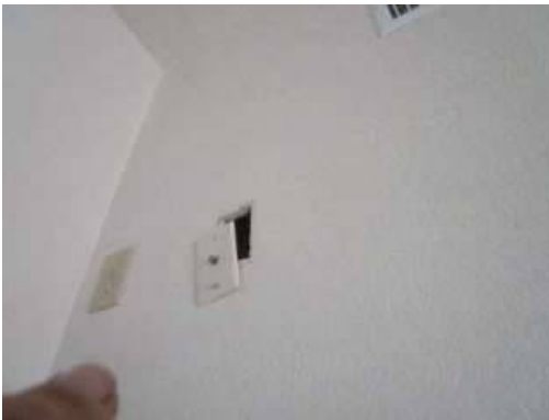
Photo 13-8 The bedroom cable cover is coming off this should be repaired.
