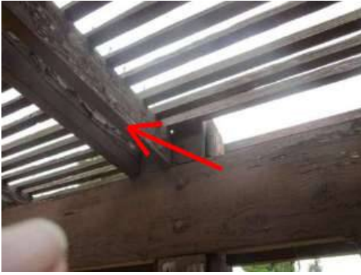
Photo 1-15 Patio cross members are deteriorating
