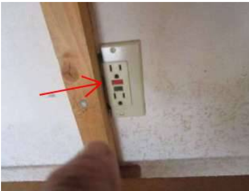
Photo 5-6 The garage GFCI plate has been cut, this is not to code, repair.
