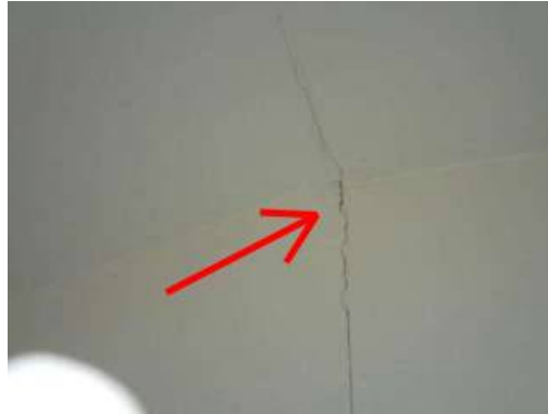
Photo 13-20 The living room wall has a crack in it and this should be evaluated by a licensed general contractor.
