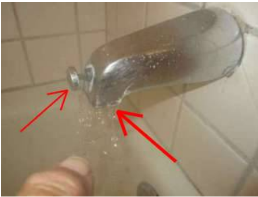
Photo 12-1 The bathtub water diffuser is broken, does not allow water to flow freely, nor does it reroute water to the shower head correctly.
