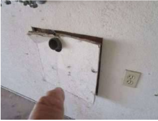
Photo 8-1 Laundry room in the garage wall needs to be repaired.
