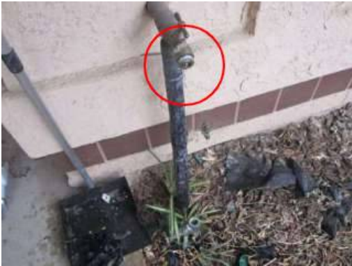
Photo 1-3 Hose bib pipe valve needs replacing
