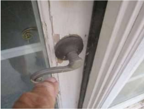
Photo 1-16 Back patio door latch does not work properly
