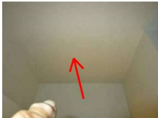
Photo 13-16 Smoke detectors need to be installed in each room. A carbon monoxide detector is missing and needs to be installed
