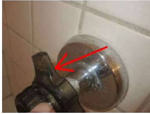
Photo 11-8 The shower valve does not turn properly, the valve is frozen.
