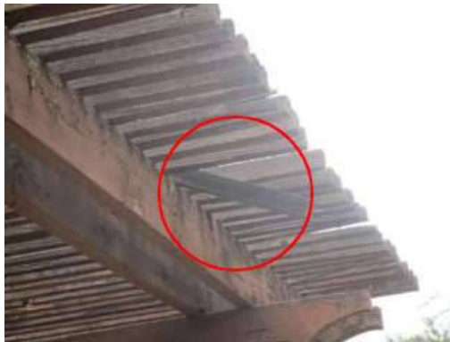
Photo 1-14 Broken lattice members around patio structure
