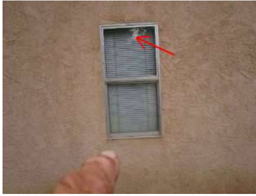
Photo 1-10 Missing window screen
