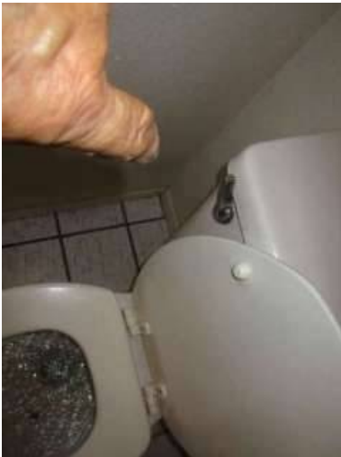
Photo 11-5 The hall bathroom toilet latch needs repair.
