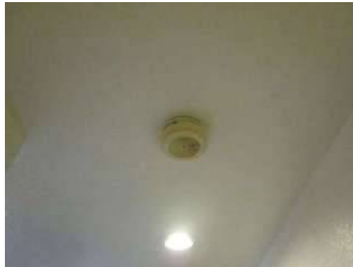
Photo 14-2 The smoke detector in the hallway appears to work.
