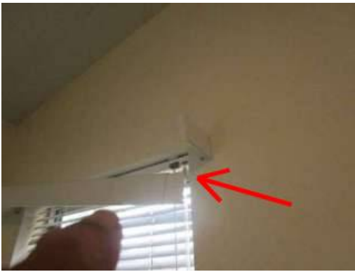
Photo 13-11 Some of the blinds need repair.
