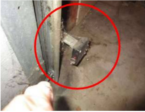
Photo 3-6 Garage door auto light sensor does not work correctly, does not allow the door to stay down, intermittent
