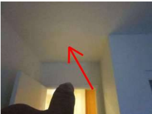
Photo 13-15 Smoke detectors need to be installed in each room. A carbon monoxide detector is missing and needs to be installed
