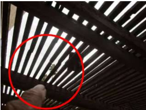
Photo 1-13 Patio lattice work has deteriorated and should be replaced
