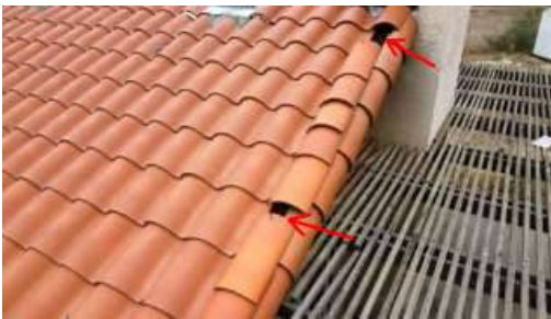
Photo 2-6 Roofing tiles have slipped or are broken in a few different areas. A licensed roofer should evaluate and repair all issues, you may want to get a roof certificate.
