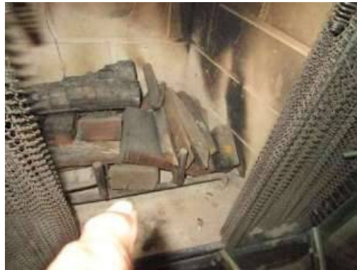
Photo 9-2 Wood burning gas fireplace. This is not an issue, just an observation.
