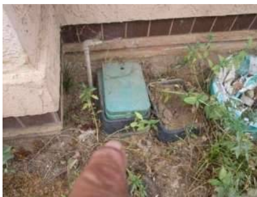
Photo 1-28 Landscaping, many of the valves are broken and do not work correctly. Entire landscaping water system needs to be repaired
