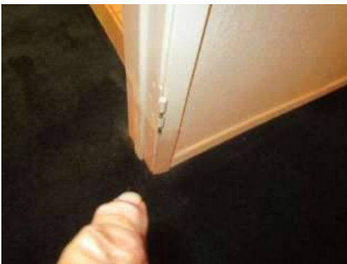
Photo 13-10 The door is missing from the closet.
