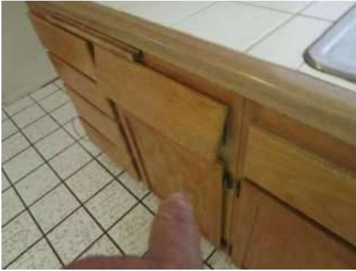
Photo 10-7 Some of the kitchen cabinet doors and drawers have defects, they should be evaluated and repaired.
