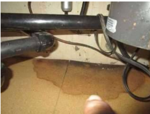
Photo 10-11 Under the kitchen cabinet sink shows signs of previous water damage this should be evaluated by a licensed plumber.
