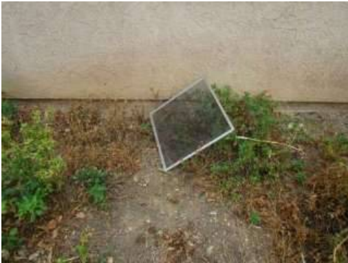
Photo 1-11 Screen is on the ground needs to be replaced
