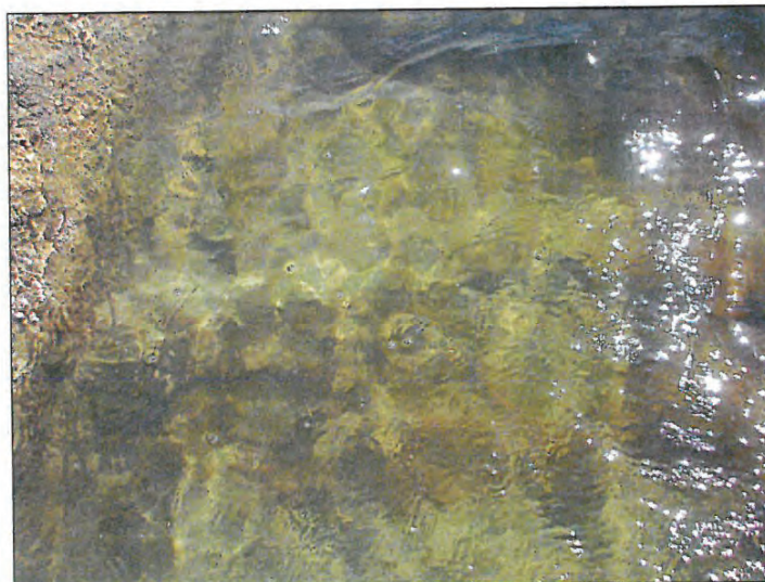
Photo #11 – Hooker Lake Dam (deteriorated spillway) (May 20, 2009)
