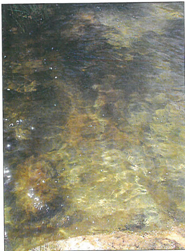
Photo #10 – Hooker Lake Dam (deteriorated spillway) (May 20, 2009)
