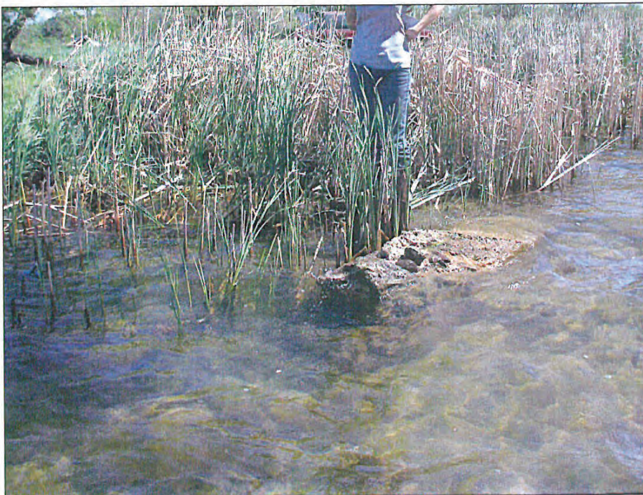
Photo #9 – Hooker Lake Dam (deteriorated left abutment) (May 20, 2009)
