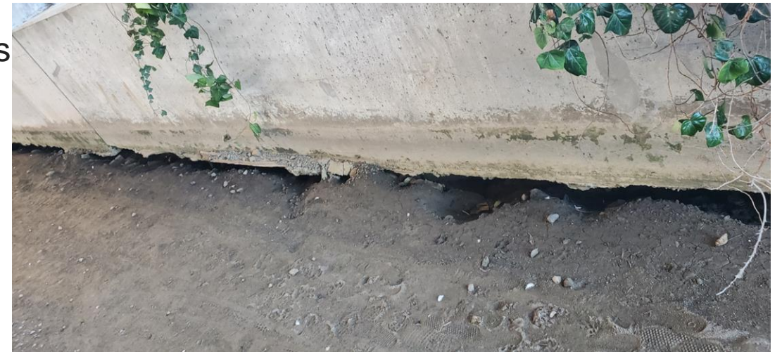
Richardson Bay Bridge Pile Cap and Settling
