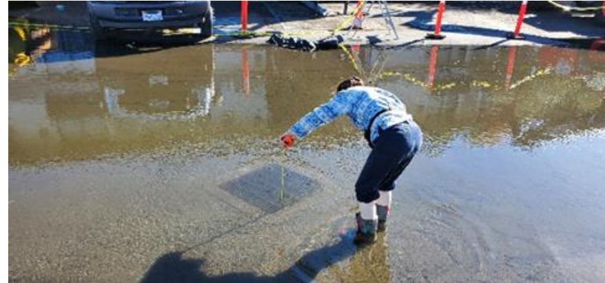
During Drainage Backflow: Height is 10-inches over grate
