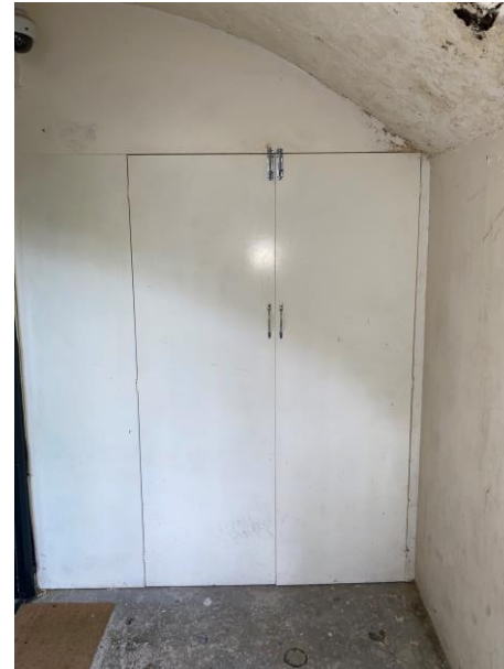
Existing LGF Gas Meter Cupboard [before]
