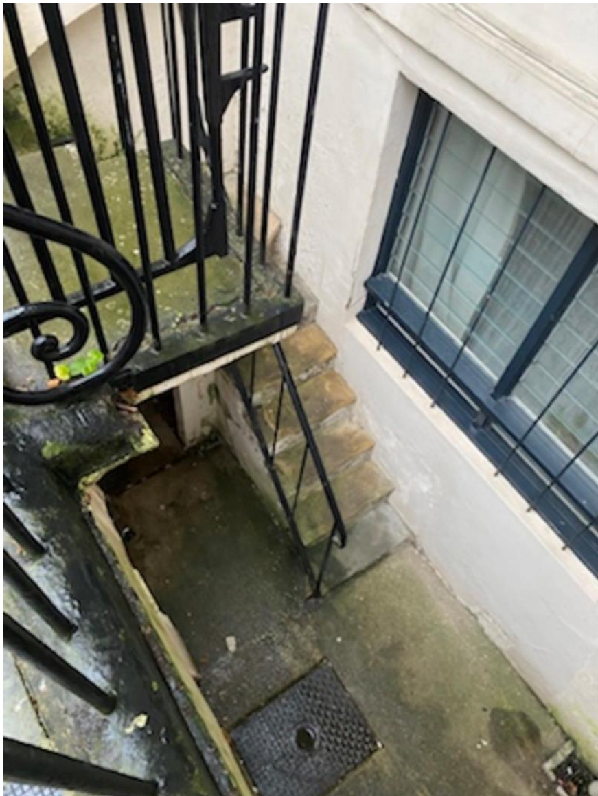
Dilapidated Unsupported LG Steps [before]
