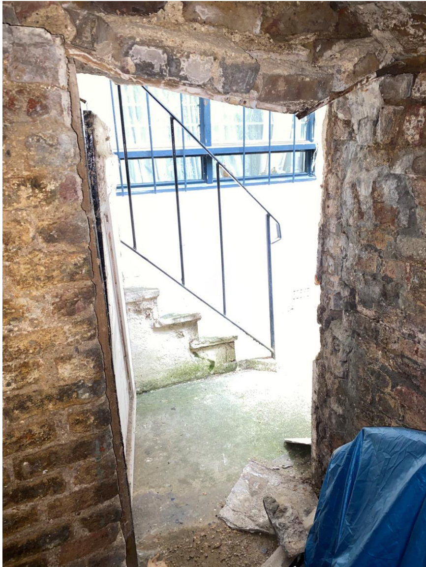
Collapsing Vault Lintels Internal [before]
