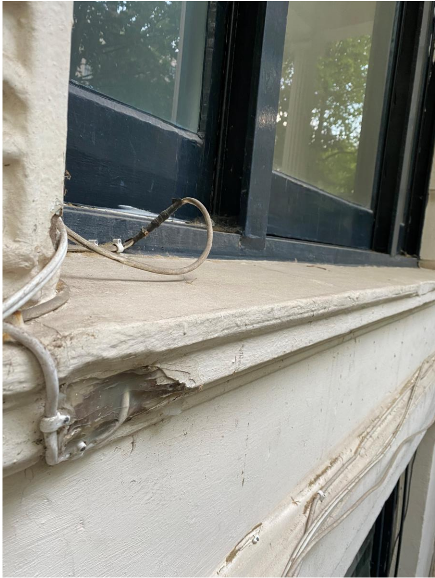
Destroyed Listed Sill Detail [before]
