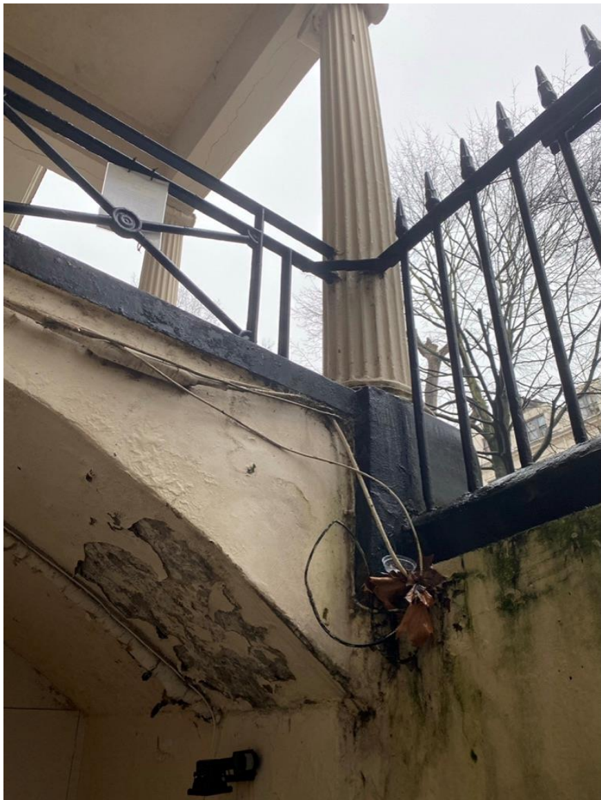
Dilapidated Unsupported Underside Portico [before]
