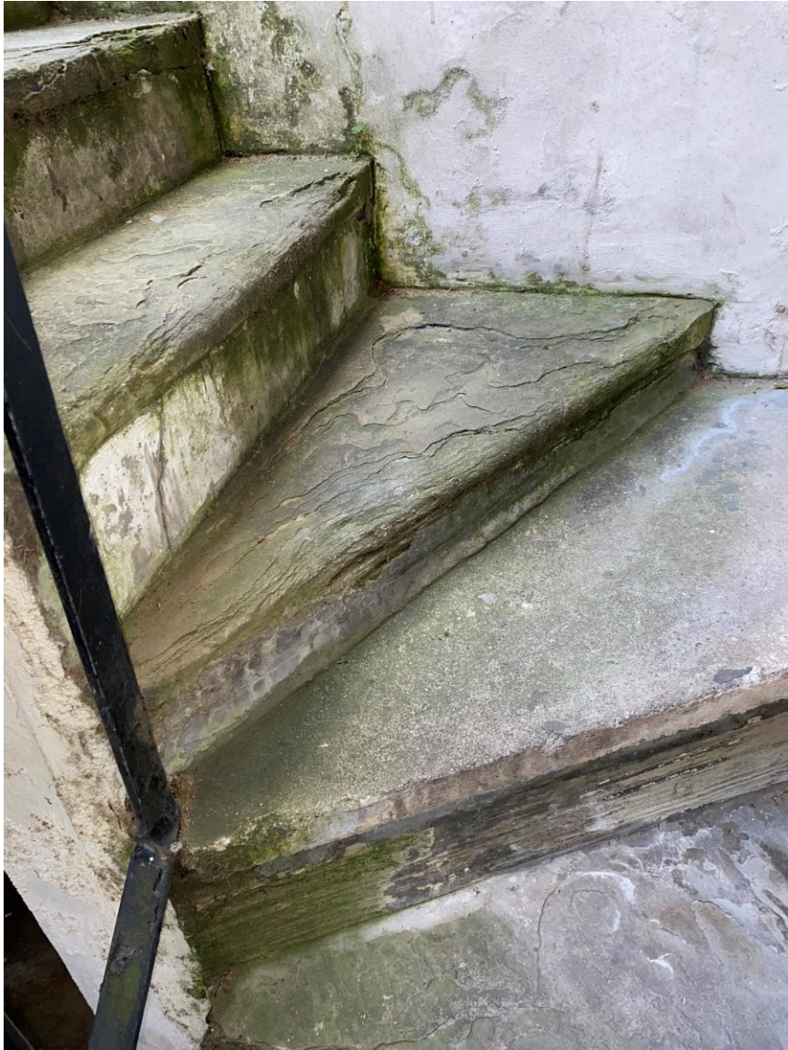
Collapsing Steps [before]
