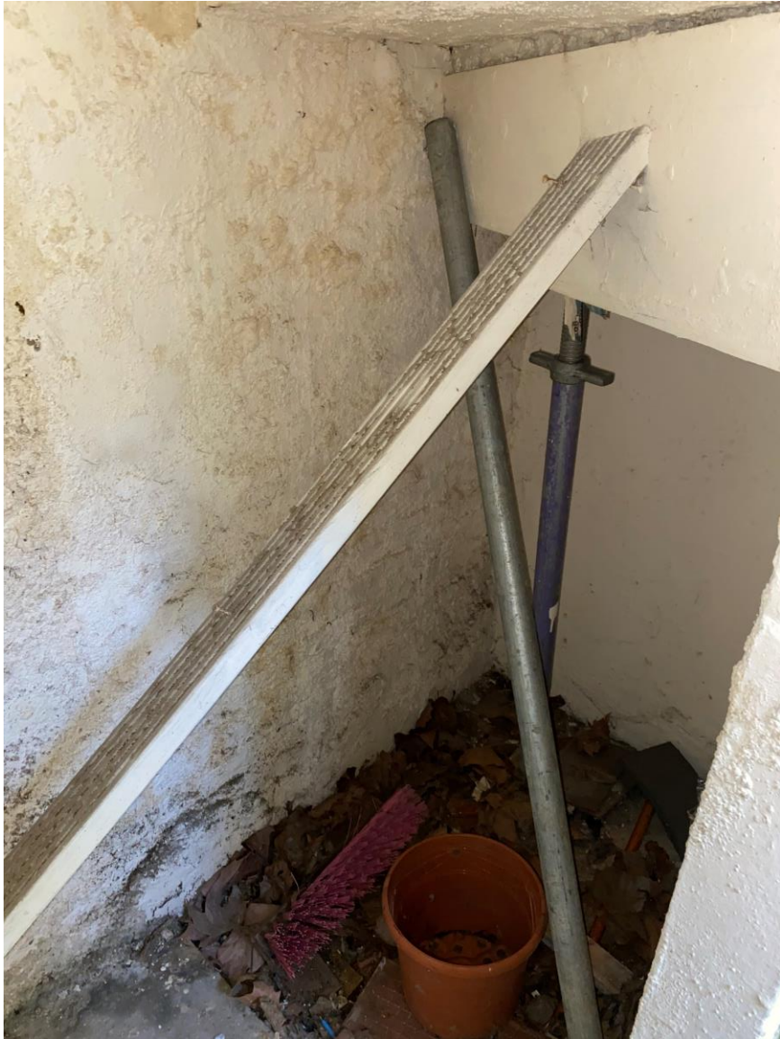
Collapsing LG Steps [before]
