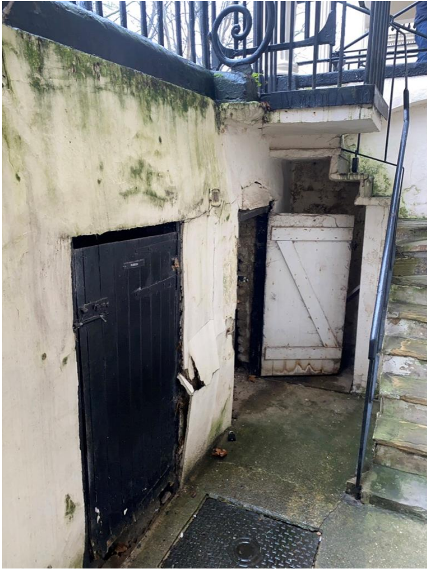
Dilapidated External Vaults Collapsing Supporting Walls & Steps [before]
