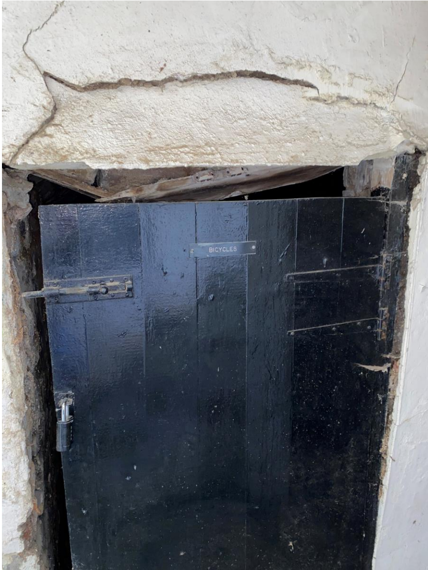
Collapsing Vault Lintels External [before]
