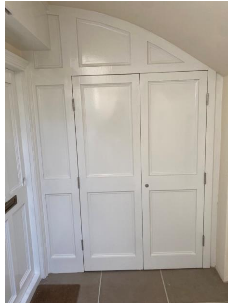
Existing LGF Gas Meter Cupboard [finished]
