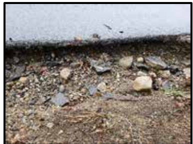
Flood Water & Damage 2023
