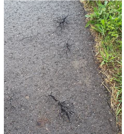
Figure 1 – “Pop-outs” caused by vegetation growing up through the trail bed. Issues like this will often require cutting out the damaged area, rectifying the underlying issues, and patching.
