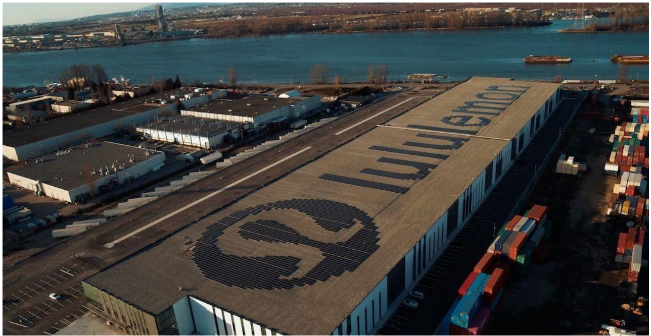
Completed solar panel system atop Lululemon's distribution centre in Delta. (Wesgroup)
