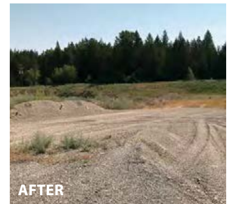
Gasoline spill cleaned up
