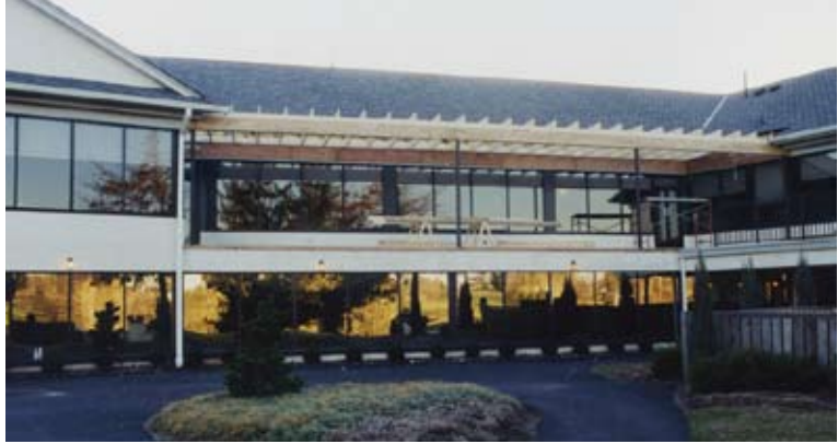
Addition #7 New roof structure being installed over the open deck as part of the Bauman addition.
