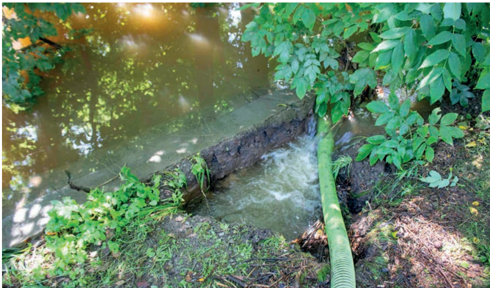
An obstructed and deteriorating culvert restricted water flow on King Street last week, contributing to severe flooding at the Legion and other nearby businesses. Letter writer Madis Tambre says the town needs to prioritize regular maintenance of its stormwater infrastructure to help prevent avoidable damage during future heavy rainfall events. FILE
