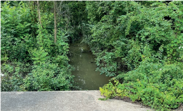
The Harrison Drain 1 on Line 6 Road shows what neglected maintenance results in — a clogged mess. BRIAN MARSHALL
