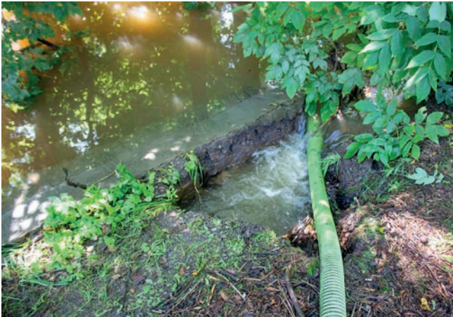
The culvert on King Street near the Legion was blocked by an obstruction Sunday, leading to water backing up and flooding nearby buildings. RICHARD HARLEY
