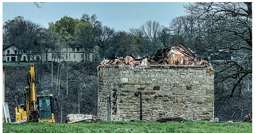
Benny Marotta is facing new heat from the town after illegally demolishing the roof of a historic schoolhouse building on his Niagara Parkway property. FILE
