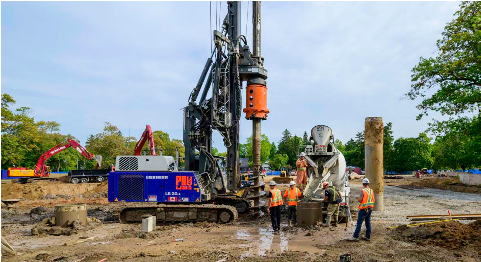
The developer of Parliament Oak has begun work without a permit and is continuing work despite a stop-work order from the Town of Niagara-on-the-Lake. Residents have complained loudly and the town will begin to enforce daily penalties. DAVE VAN DE LAAR
