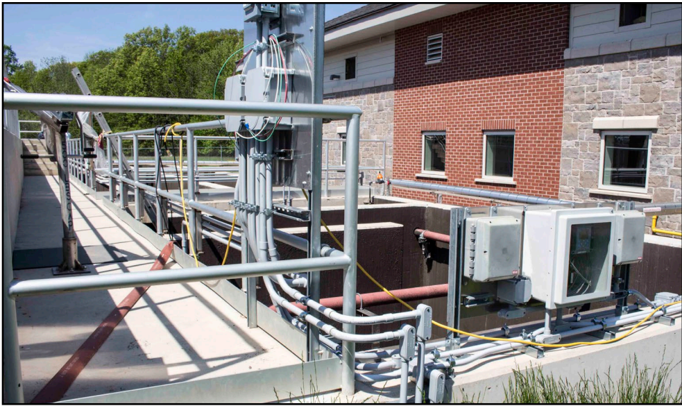
The new wastewater treatment plant on Lakeshore Road is expected to open in August. (Richard Harley)
