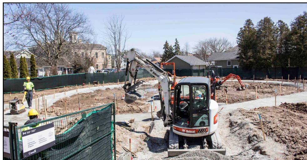
Construction being done at the future Voices of Freedom Park on Regent Street. (Richard Harley)
