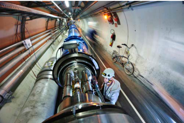
A close-up of the superconducting magnets lining the LHC tunnel, hinting at the sheer engineering power and precision behind particle acceleration — the backbone of modern experimental physics. SOURCED
