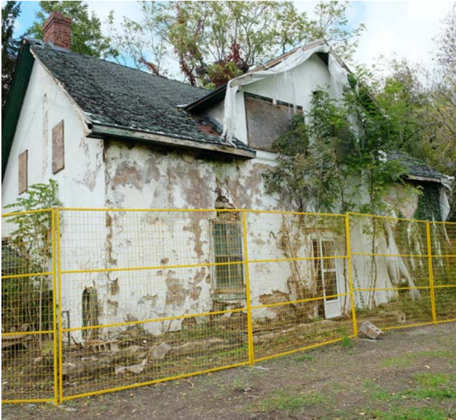
The 266-year-old David Secord House is in a state of disrepair. But developer Rainer Hummel hopes to save it.
