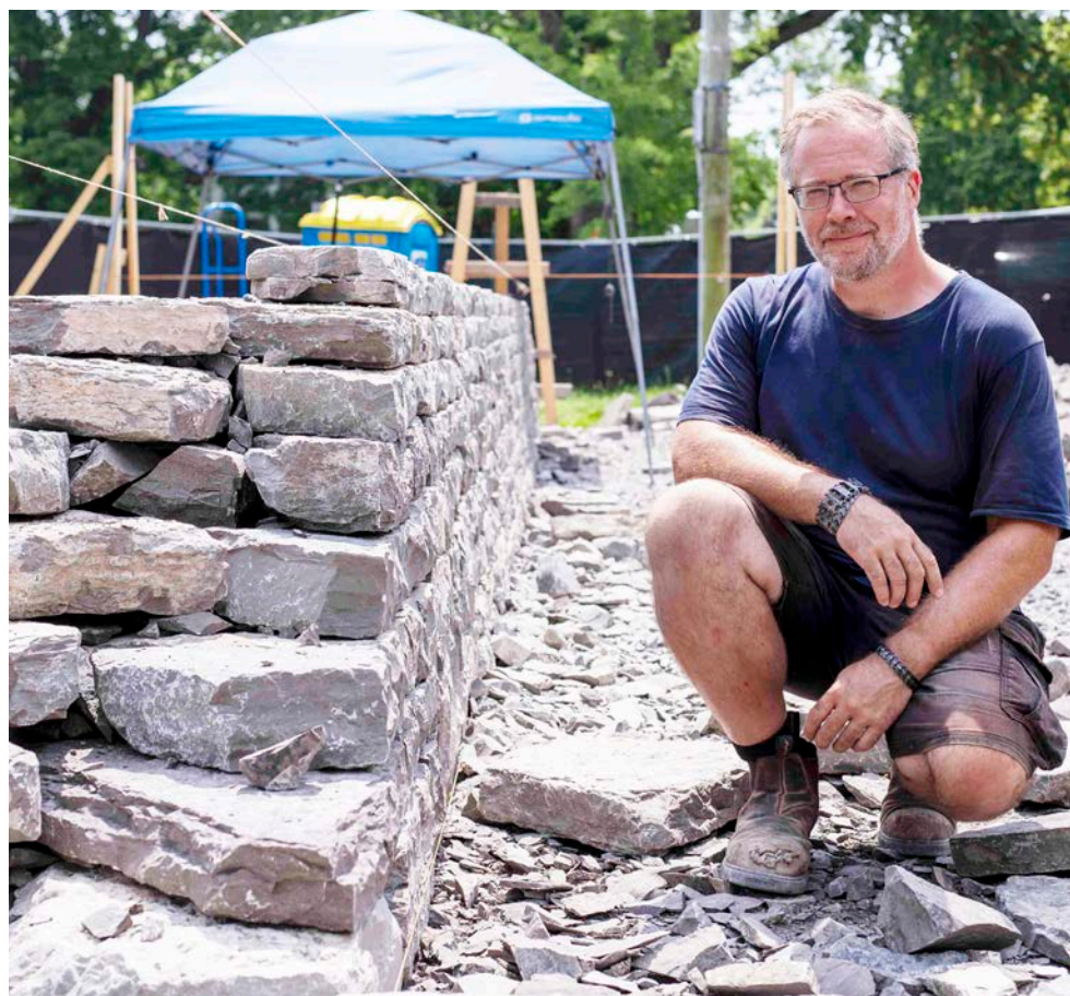
Menno Braam's drystone wall will be about five feet high when completed. EVAN LOREE
