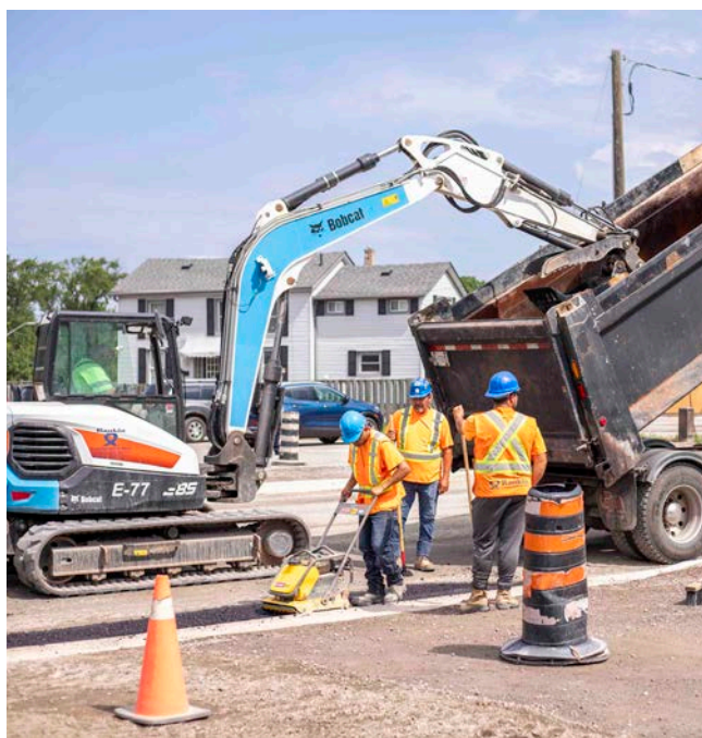
Construction crews started paving a portion of Niagara Stone Road on Wednesday. MADDY GORDON
