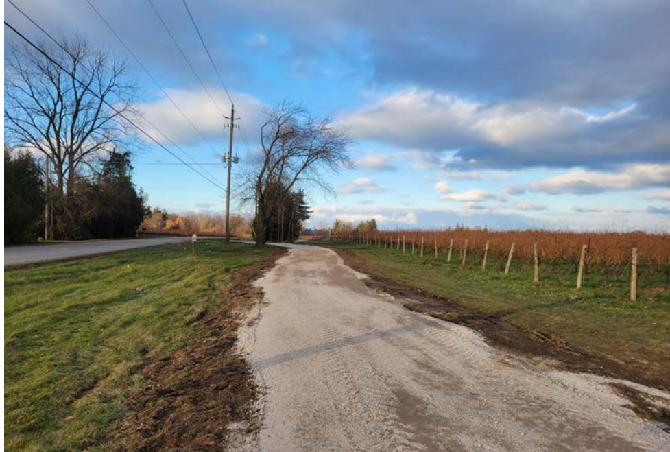
Work on phase two of the heritage trail began in November 2023 and should be completed up to Line 3 Road later this year. TONY CHISHOLM
