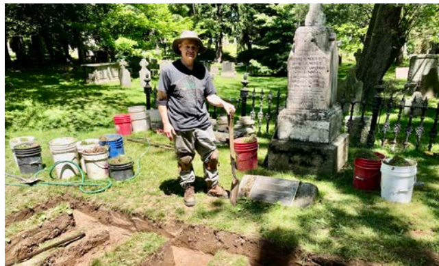
The Royal Canadian Yacht Club plot at St. Mark's cemetery is undergoing a major restoration by Alan Ernest and his team from Carlisle. ROSS ROBINSON
