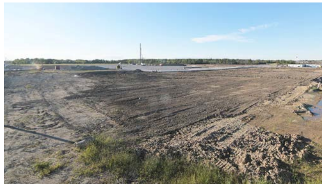
Work is underway at the site of the new South Niagara Hospital site in Niagara Falls. SUPPLIED/NIAGARA HEALTH
