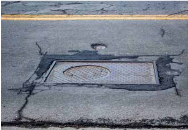
A loose grate on Mississagua Street is giving neighbours a headache. RICHARD HARLEY
