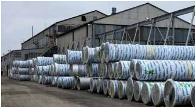
For the first time, the Port Weller drydock is also completing non-marine work, assembling wastewater outfall pipes to be used in the new Ashbridge's Bay Wastewater Treatment Plant in Toronto. The pipes are shown here, prior to final assembly. TIM TAYLOR
