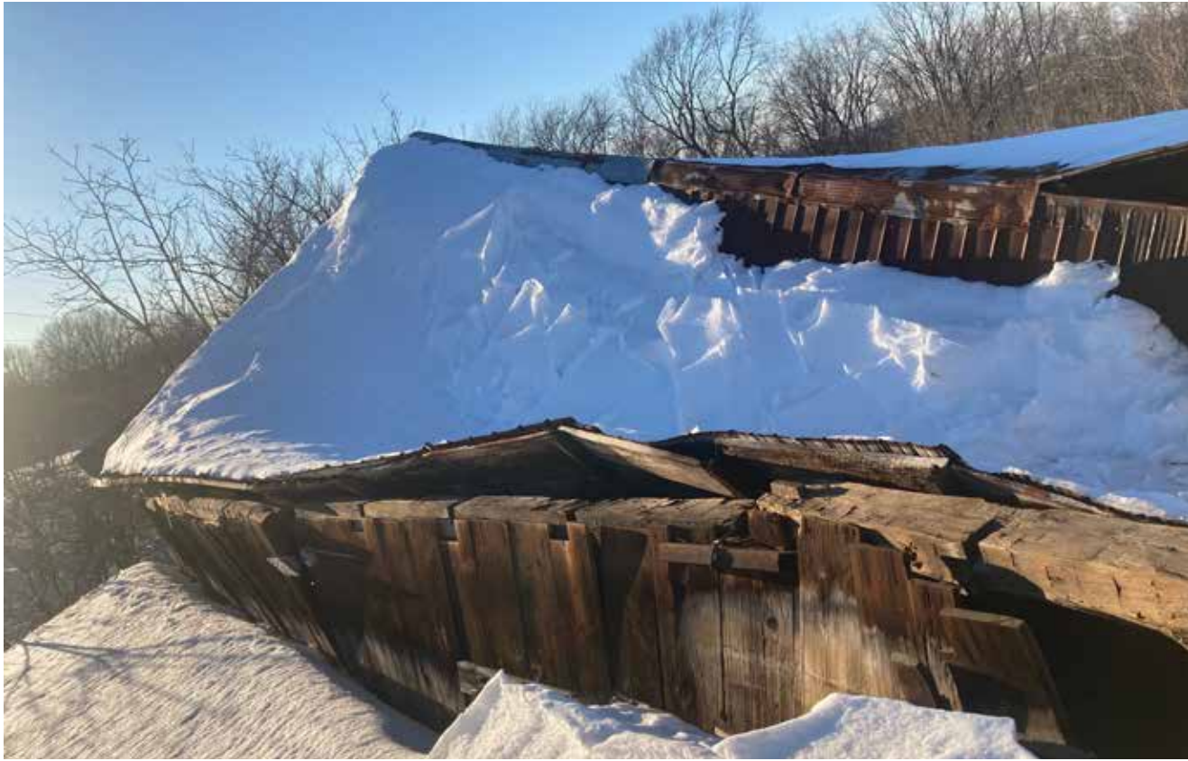
Dinah McGibbon’s barn roof collapsed after a series of heavy snow storms. She is trying to raise money to help with the repairs, which she said will be financially crippling. SUPPLIED
