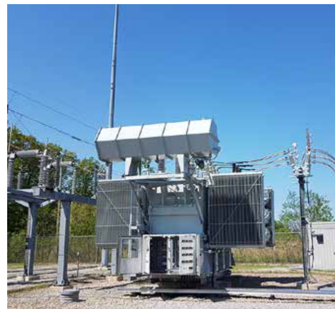
A new 83 MVA transformer has been installed at NOTL Hydro's York Road station. SUPPLIED
