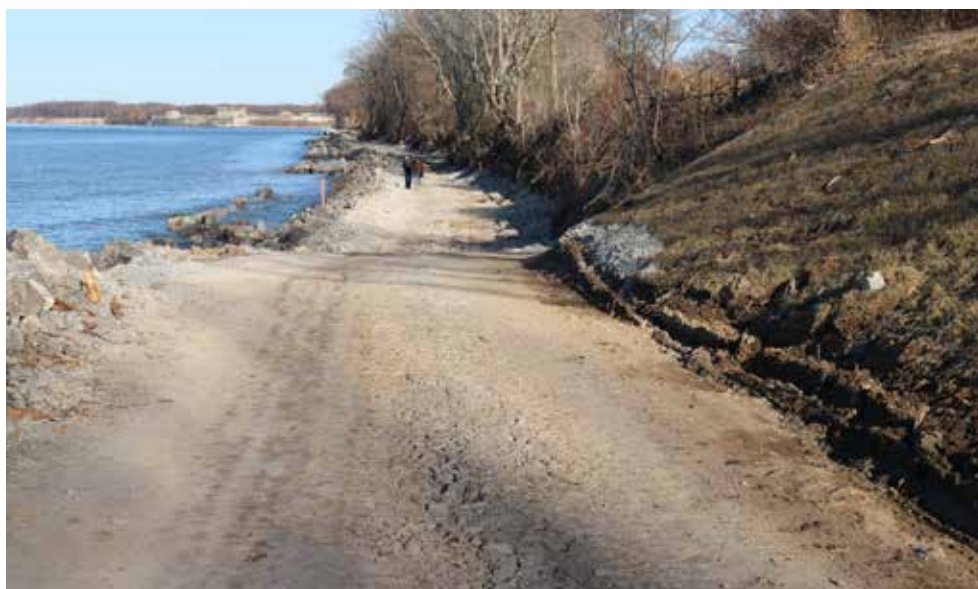
Large stones are dumped into Lake Ontario to improve shoreline protection along the waterfront at the Niagara Golf Club. DARIYA BAIGUZHIYEVA
