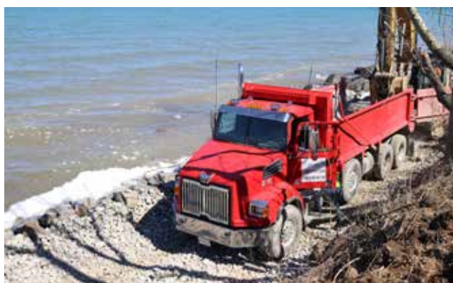
A truck carries large stones to be used for shoreline protection along the waterfront at the Niagara Golf Club. DARIYA BAIGUZHIYEVA
