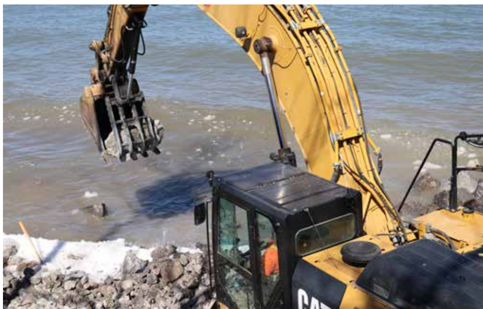
Large stones are dumped into Lake Ontario to improve shoreline protection along the waterfront at the Niagara Golf Club. DARIYA BAIGUZHIYEVA
